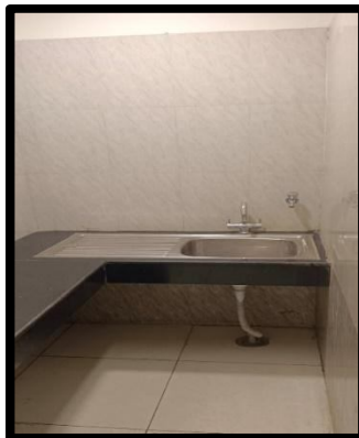
Kitchen with RO Water
