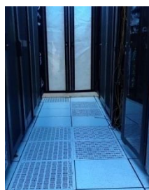
Pic: Server Room
